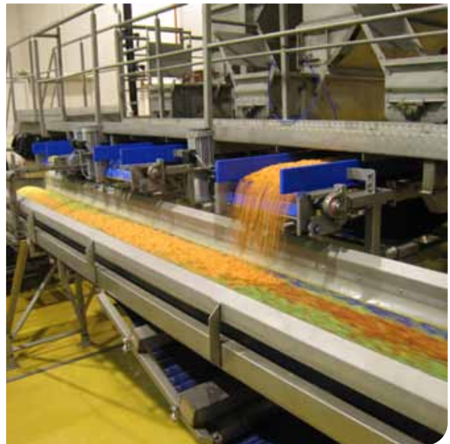
▲ Installations in food processing lines
